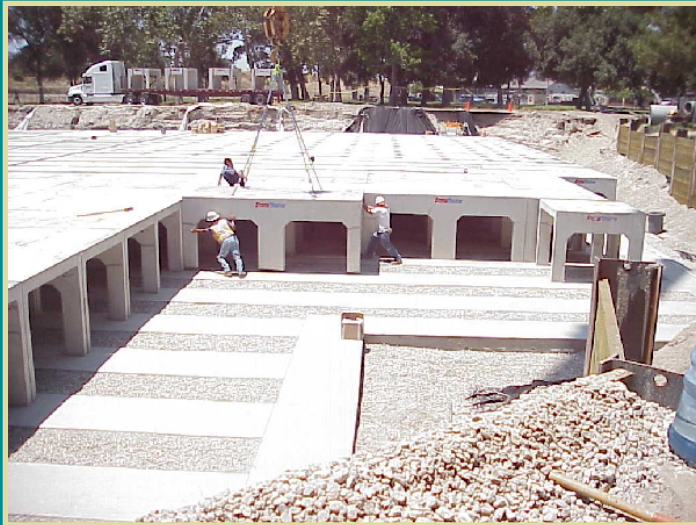
Underground Infiltration Chambers
