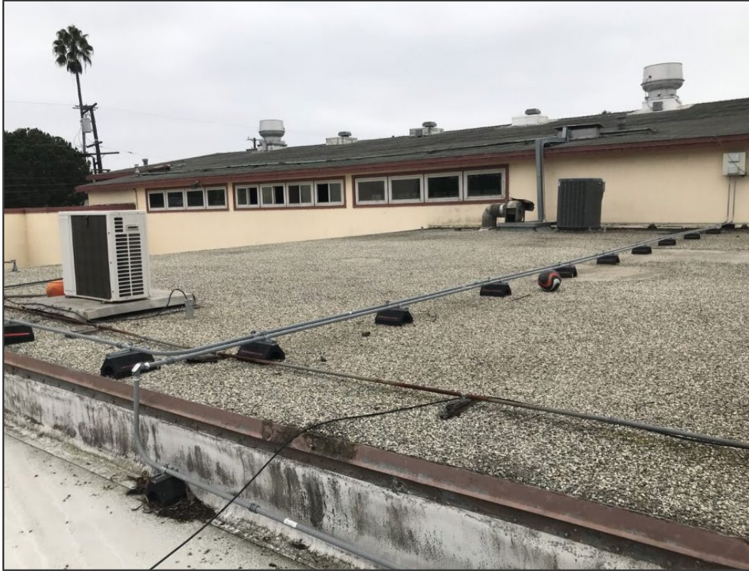
Figure 10 Existing Mix of Roof- White Roof, Built up with Gravel and Asphalt Shingles
